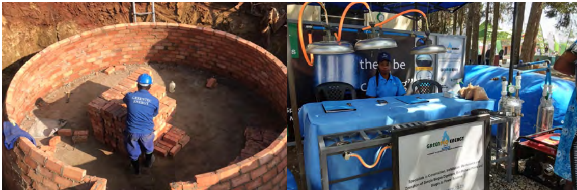
▶ A GreenTEC Energy biogas mason works on a fixed dome biogas plant in Bulawayo
